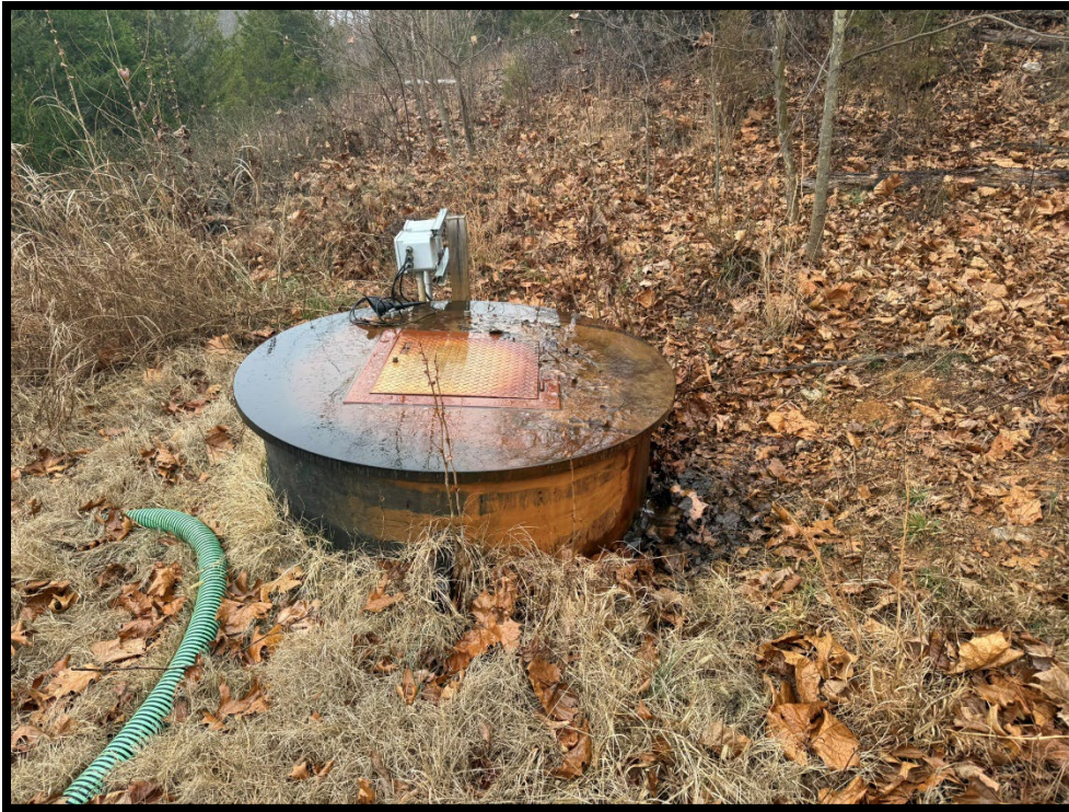
Photograph 3: View of VLCS-1 overflowing.
